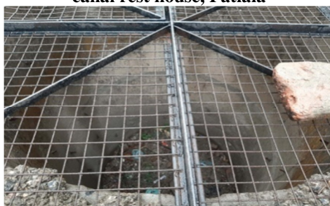
Artificial recharge structure at Dhangeria canal rest house, Patiala
