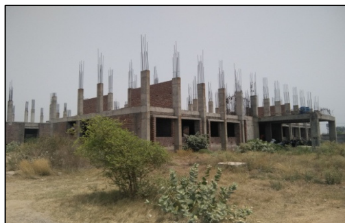
Incomplete MSDC building at Amritsar, as on 24 May 2018
