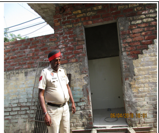
Non-functional toilet at Police Post, Shivala, Amritsar (06-04-2018)
