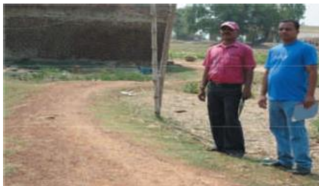
Photograph showing sub-standard Earthen- murram road at Pakur district Hiranandpur GP
