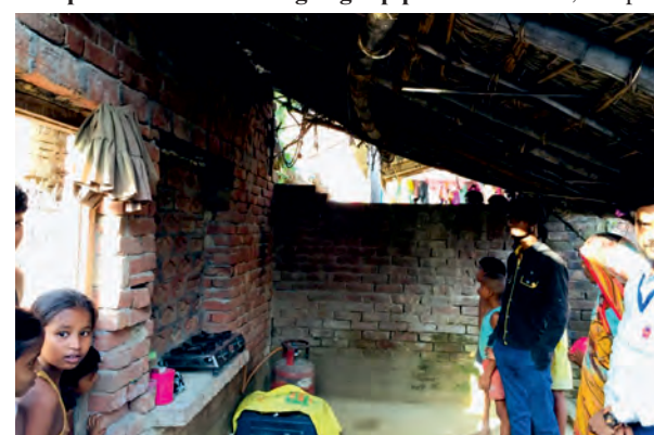
4. LPG connections installed in hay roof: HPCL, Sitapur
