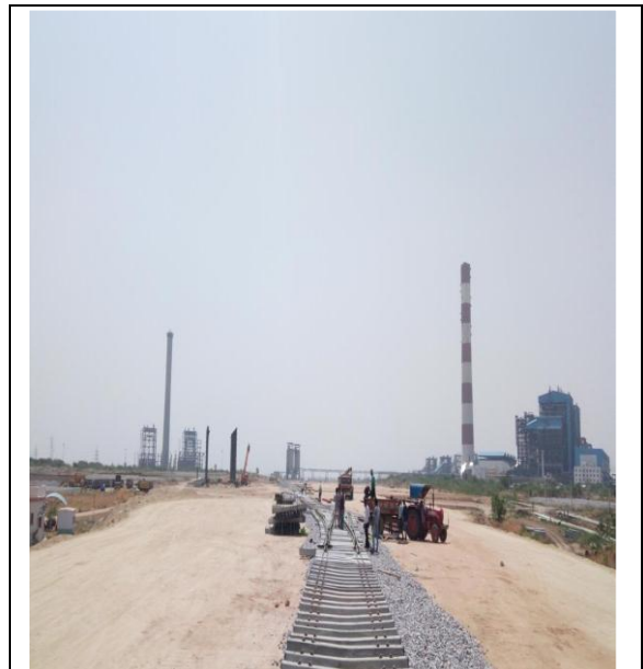
Picture No. 2.1.2: Track laying in RSMY works Source: Monthly Meeting Reports of the Management of April 2018
