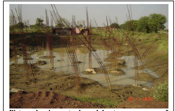
Picture showing water logged due to non progress of work and column steel has rusted at Mathpurena site - BSUP Raipur
