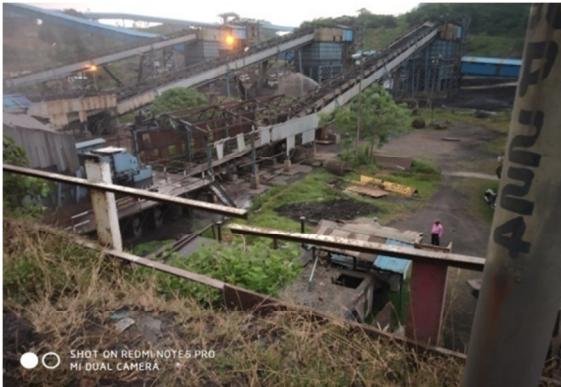
Pic. 01: Para No. 4.6.1, Table No. 06, Sl. No. 01: Un-covered conveyor belt at CHP in Lingraj Mine of MCL
