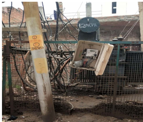
Meter installed at Distribution Transformer under EDD, Chibramau not connected to modem
