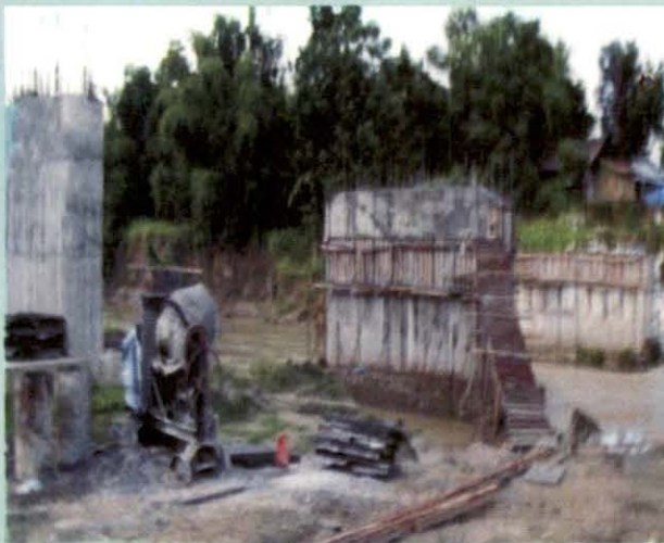
A photograph of incomplete bridge on "Road from Purana Bazar (NH 39 By pass) to Kohima-Bokajan" (October 2008).
