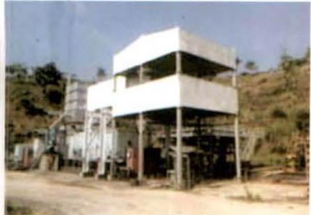
Generating Unit Ph-III of Rokhia (Tripura)
