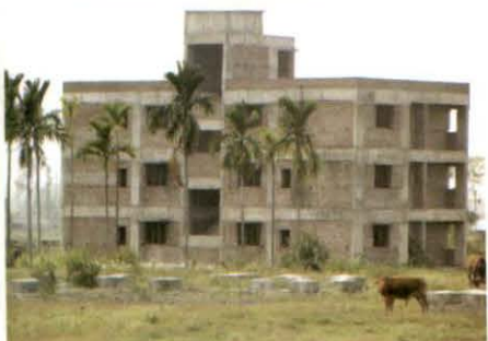
Idling of Building-of 22.92 MW HFO based thermal Power Plant at Dimapur (Nagaland)
