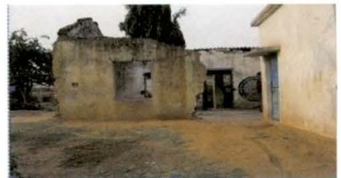
Dilapidated building of AWC Marjadapur
