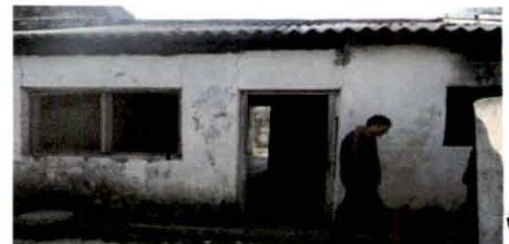
Ghantapada S.C in dilapidated condition
