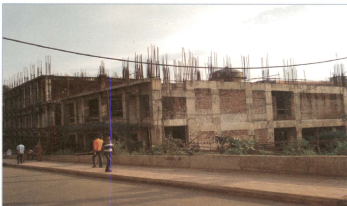
Incomplete teaching block at GBP Hospital, Agartala scheduled to be completed in December 2007
