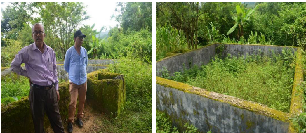
Filter Media (left) and Settling tank (right) overgrown with grasses
