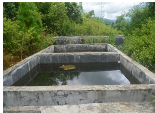
Distribution pipelines not executed even after three years from the stipulated date of completion
