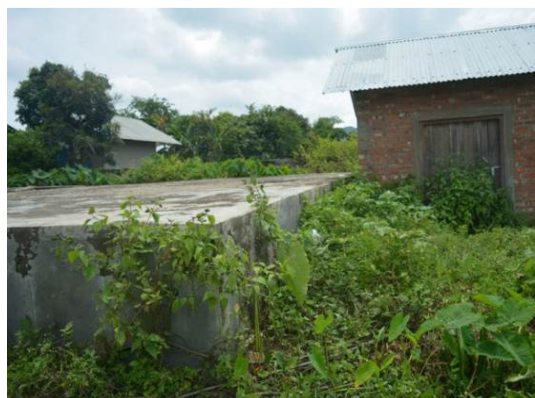
Reservoir and Pump House for storing treated water for further distribution
