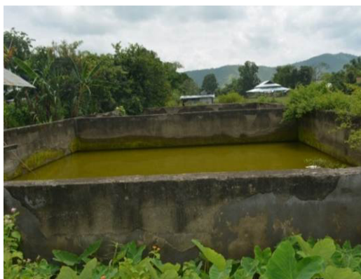
Deplorable condition of Slow sand filter for treatment of raw water
