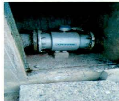
Defective flowmeter of CETP at Kanpur
