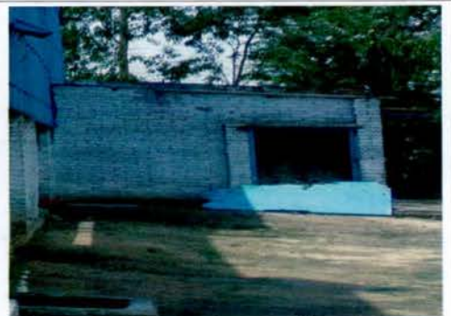
Hazardous waste storage without doors near Chak Ganjaria at Lucknow
