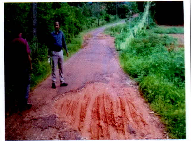
Condition of asphalted road within six months of construction in Aivathoklu village (Dakshina Kannada) (16.07.2014)
