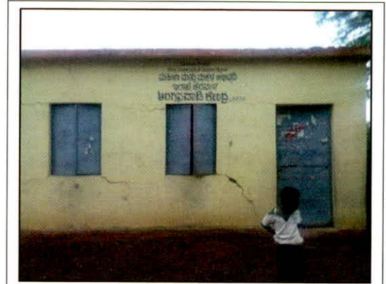
Poor quality construction of Anganwadi in Haraval village, Kalaburagi district (27.08.2014)
