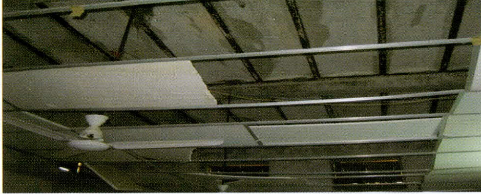
Damaged ceiling at ZP High School, Mukrambad, Nanded
