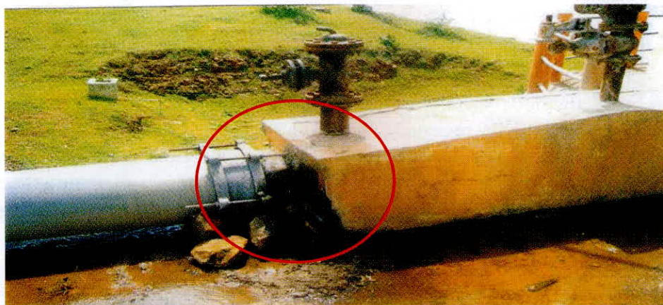
Leakages at the common head works of Lakhanwada/Deulgaon Shakharsa
