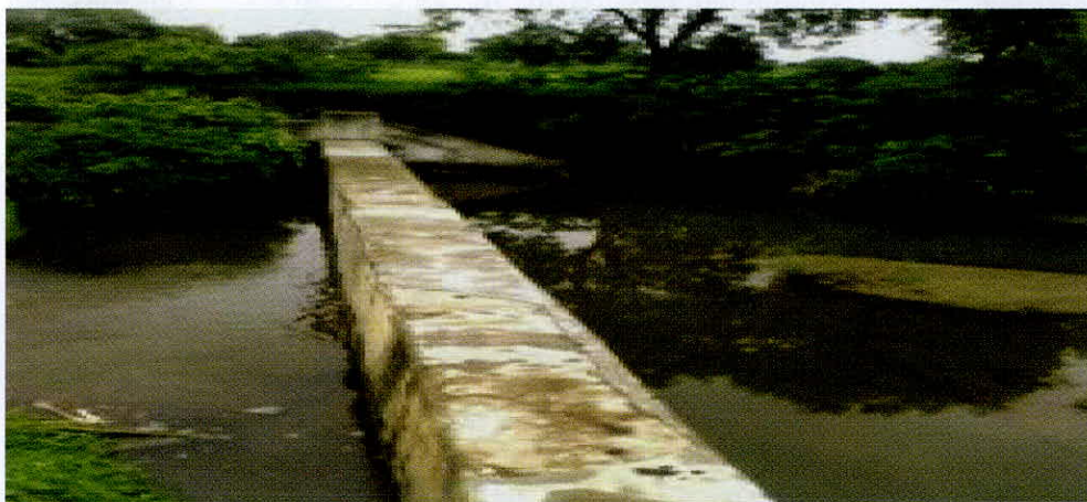
Cement nalla bund at Andhera village with heavy leakages
