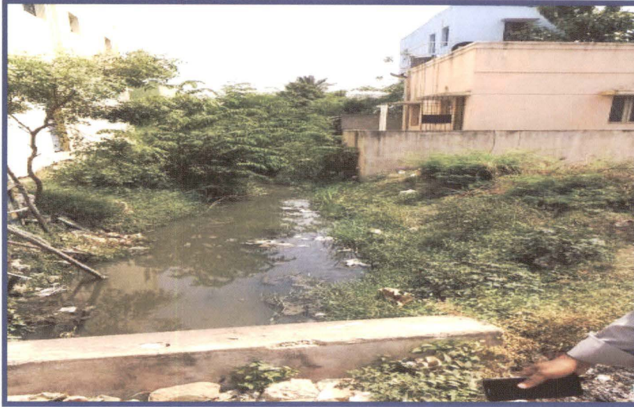
Exhibit: 2.6: Smaller than stipulated culvert at Kundrathur Village
