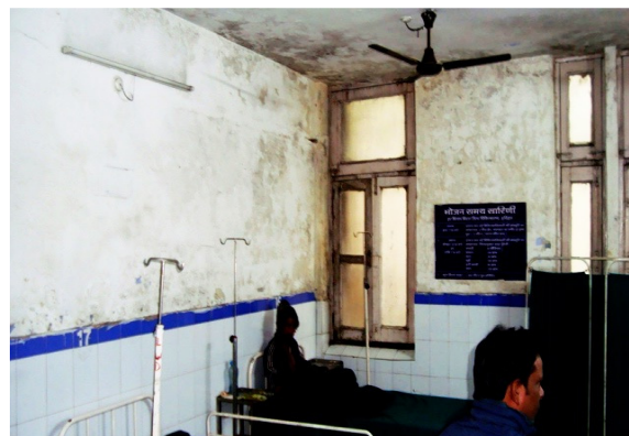
Photograph-19: Ward in dilapidated condition in DH Haridwar
