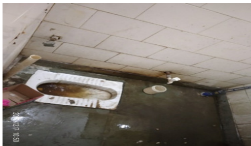
Photograph-15: Toilet in non-usable condition in JH Udham Singh Nagar
