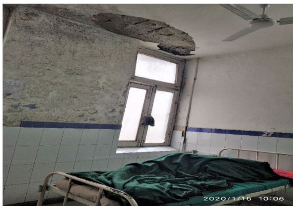
Photograph-18: Broken roof in Ward in DH Haridwar
