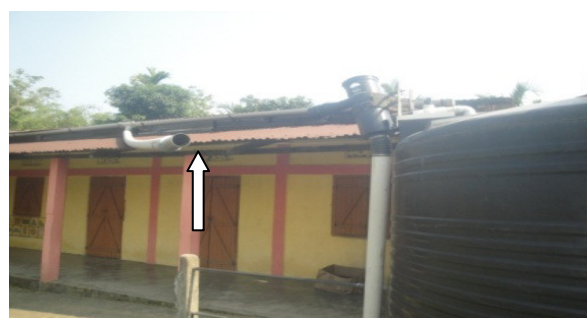
Bihara Bazar MV School under Silchar-I Division with Broken gutter pipe (12 May 2017)
