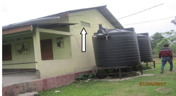
Baidyagarh Girls MES under Rangia Division with Broken gutter pipe (21 April 2017)
