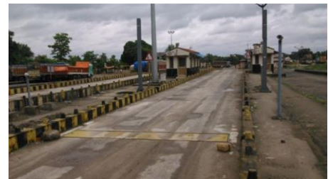
Non-functional weighbridges with damaged installations
