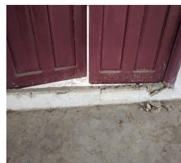
Cracks on the floor
