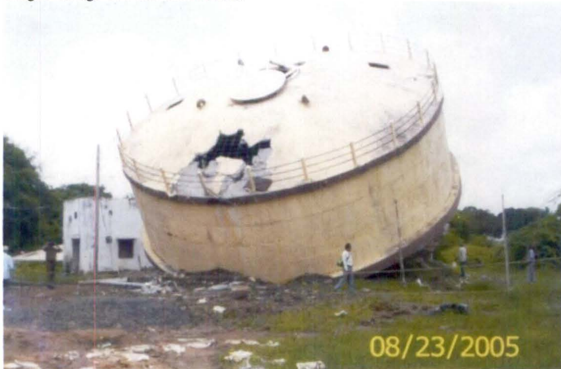
Photo showing Collapsed Elevated Storage Reservoir
