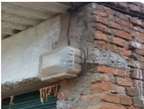
(Service cable not installed as per the provision of work order at Ambikapur town)
