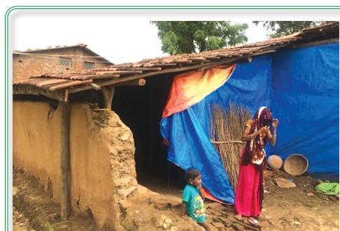
Picture 1: Dilapidated kutcha house in Piplod village, Devgadbaria taluka under Dahod district.
